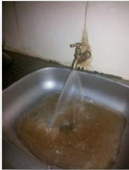
Piped water before the filters were distributed
